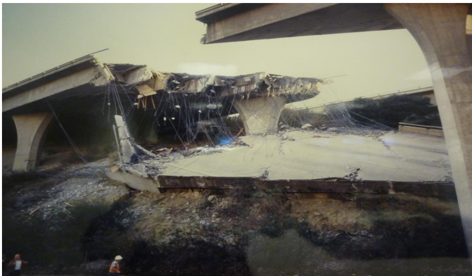
Intentional bridge explosion with multiple victims trapped
